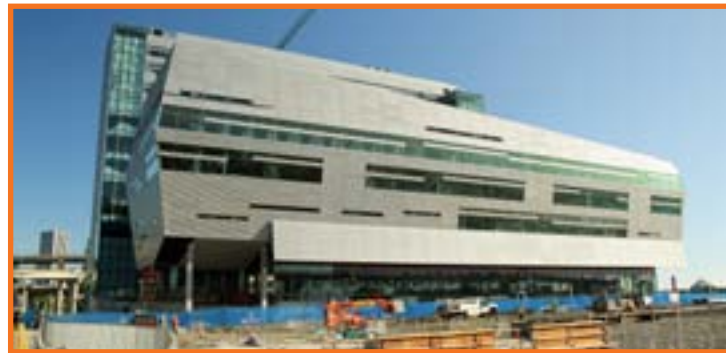
The CLSB south tower. The sloped 'ceiling' at the lower left is the floor of the College's large lecture hall.
