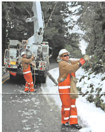
Linemen Jeff White and Scott Johnson replace power lines downed by a freak snowstorm in 2012
